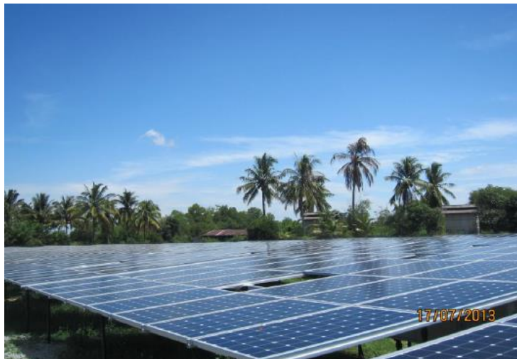
Figure 11: OCK's 1MW solar farm in Kelantan
